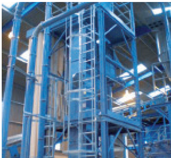
Fig. 2: Air stream separator with maintenance platform
